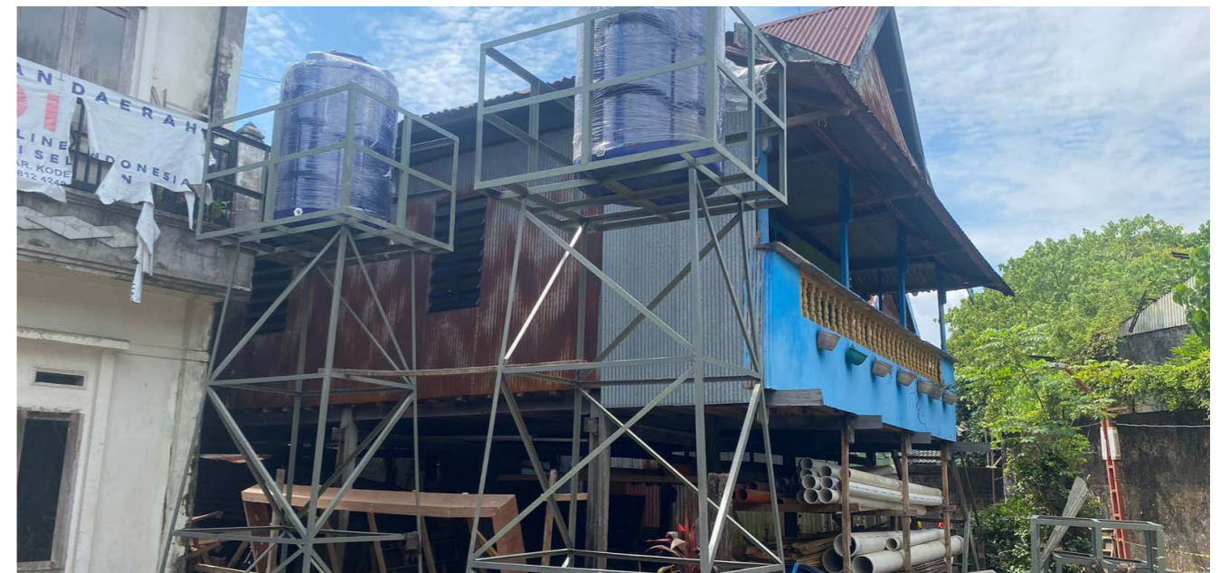
Rain water tanks
