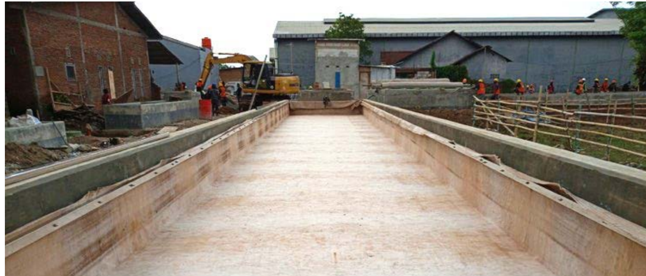
Septic tanks and wetlands
