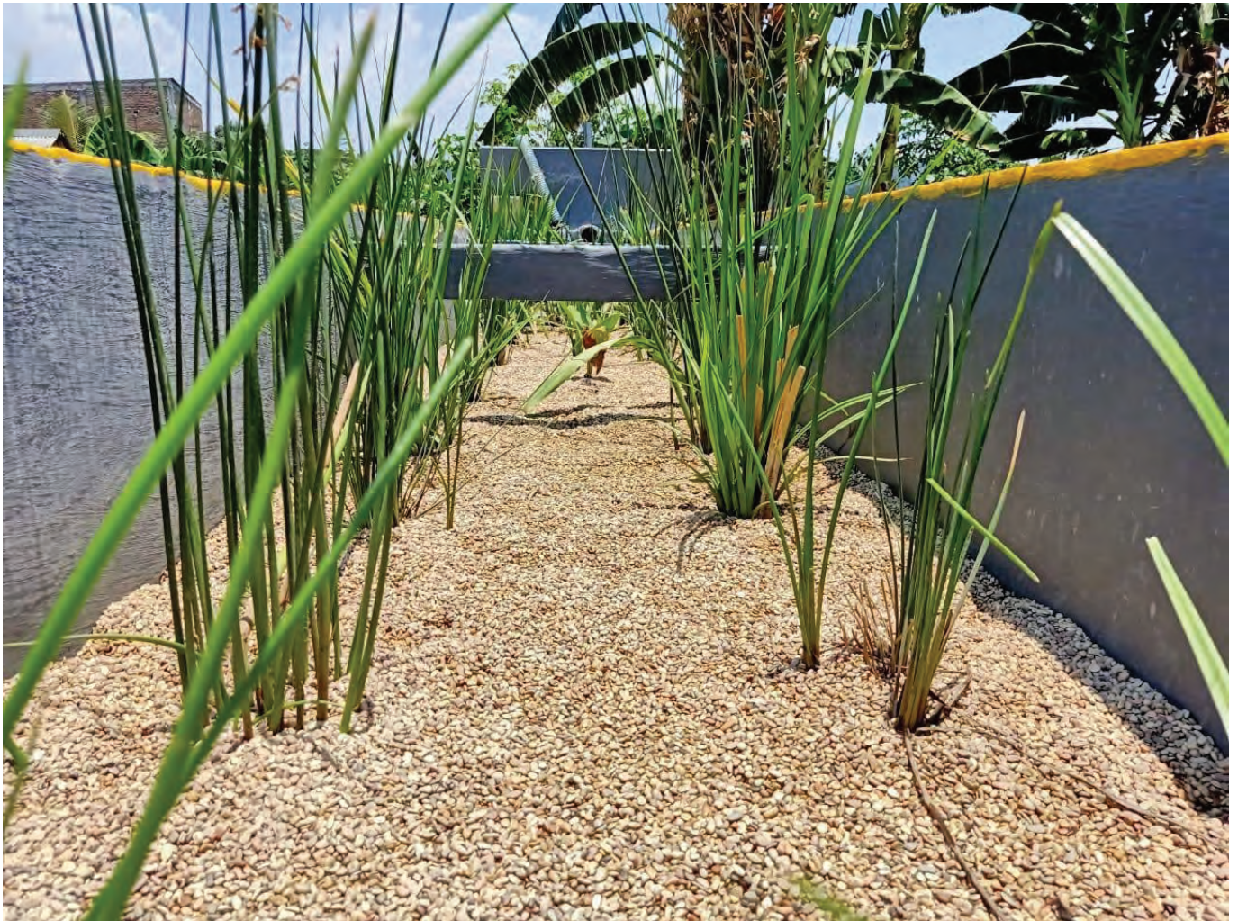
Subsurface wetland at Batua, Makassar. All effluent flows are below the surface of the gravel media and key biological treatment processes occur in the plant root zone.
