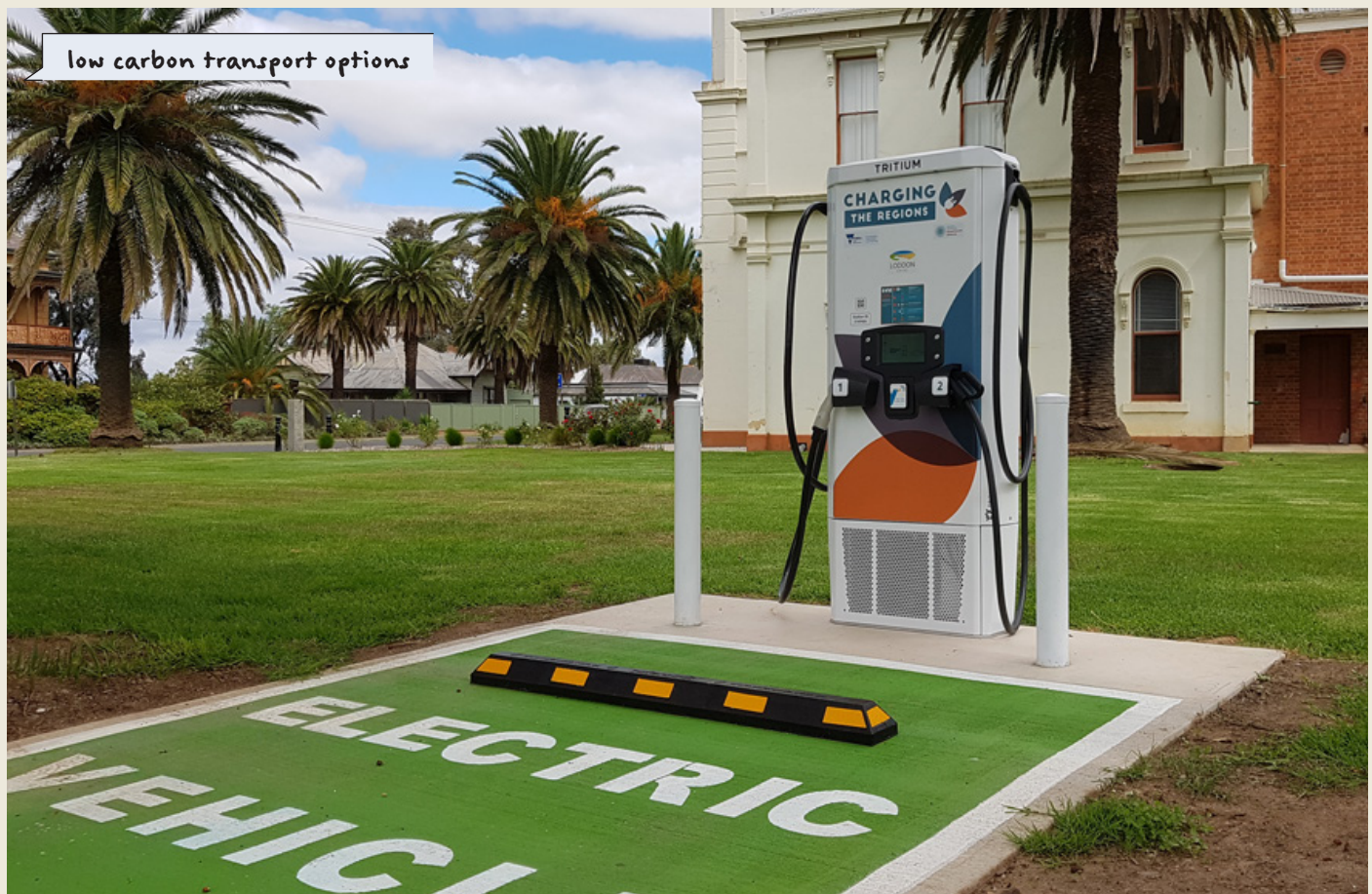
A charging station installed in Inglewood, VIC as part of the Charging the Regions Project.
