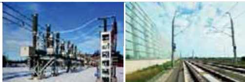
Power / Electrification Solutions
