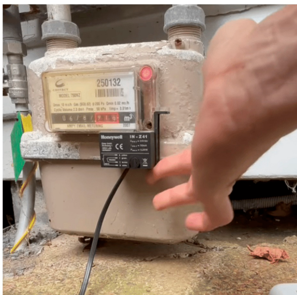
Figure 2. IN-Z41 pulse reader being connected to a gas meter (Source: Tether)
