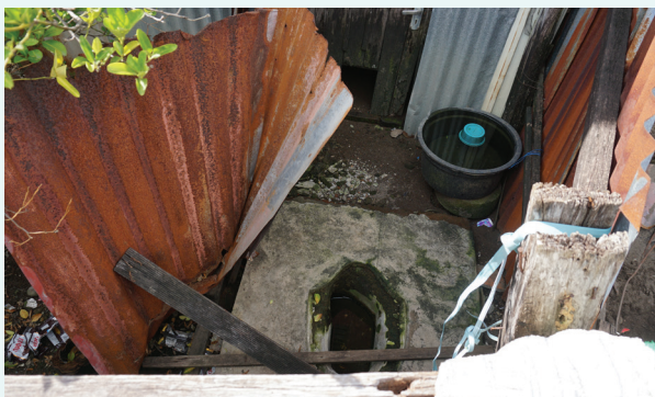
A toilet identified to be in poor condition, without walls and a roof.
