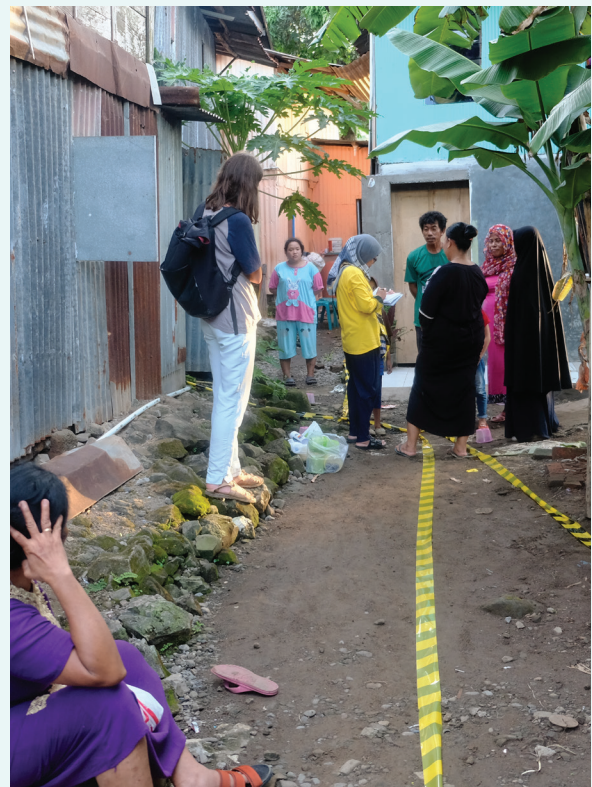
Discussing and marking connections between infrastructural elements, from private toilets to pressure pods.
