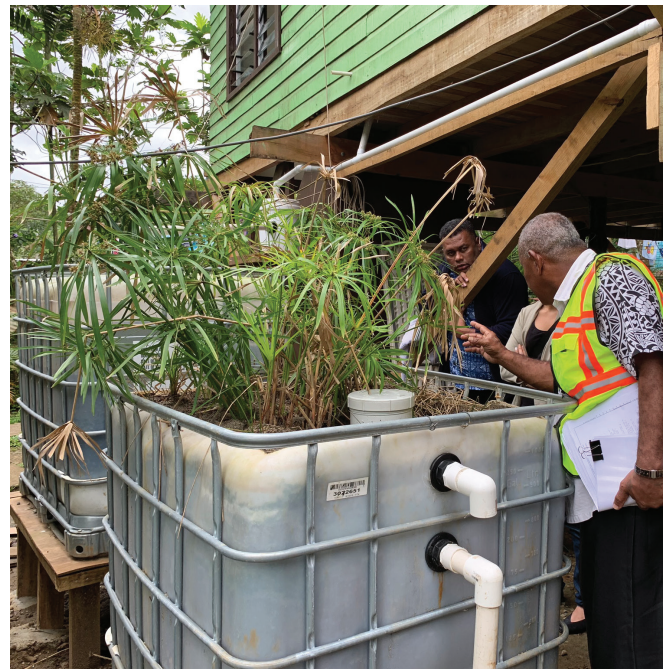
Household-scale biofilters for greywater treatment in Fiji (top) and Indonesia (bottom)
